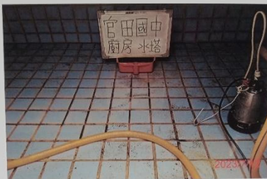
(廚房)水塔清洗前
