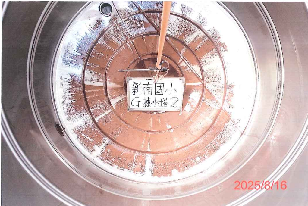
(G棟-2)水塔清洗前
