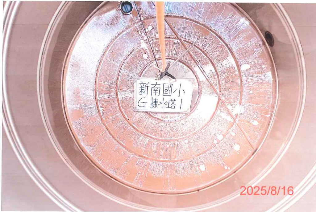
(G棟-1)水塔清洗前
